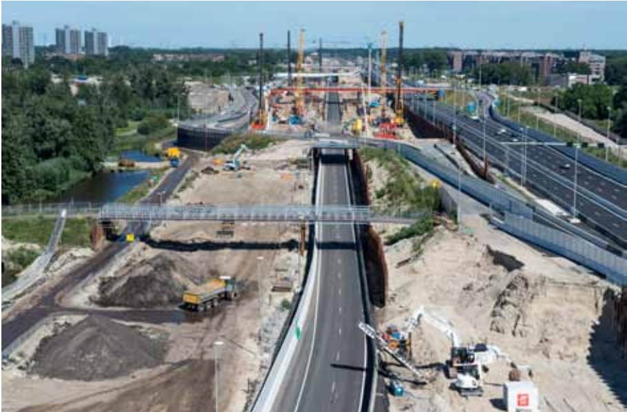
Figure 7.6: The Gaasperdammer Tunnel under construction between the De Bijlmer and Gaasperdam districts; the reversible lane in the center and the temporary A9 on the right (Photo: Rijkswaterstaat)
