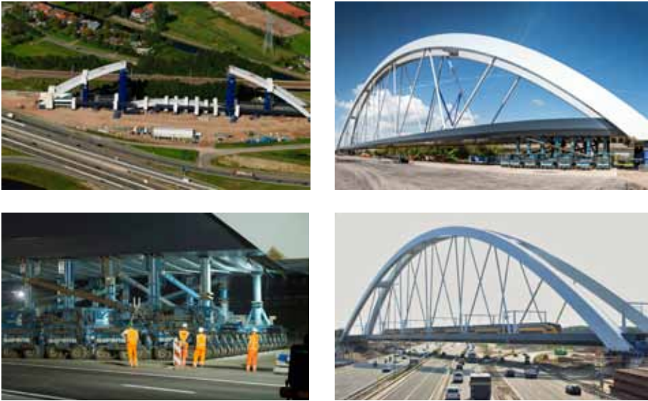
Figure 7.3: The railroad bridge over the A1 at Muiderberg: in assembly alongside the A1 (upper left), ready for transport (upper right), some of the 976 wheels under the bridge (lower left), and its final location (lower right) (Photo's: Rijkswaterstaat)
