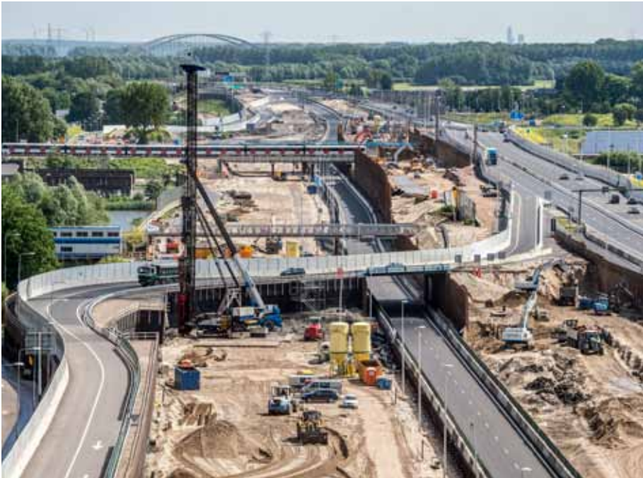
Figure 7.2: The reversible lane on the construction site of the Gaasperdammer Tunnel (Photo: IXAS)
