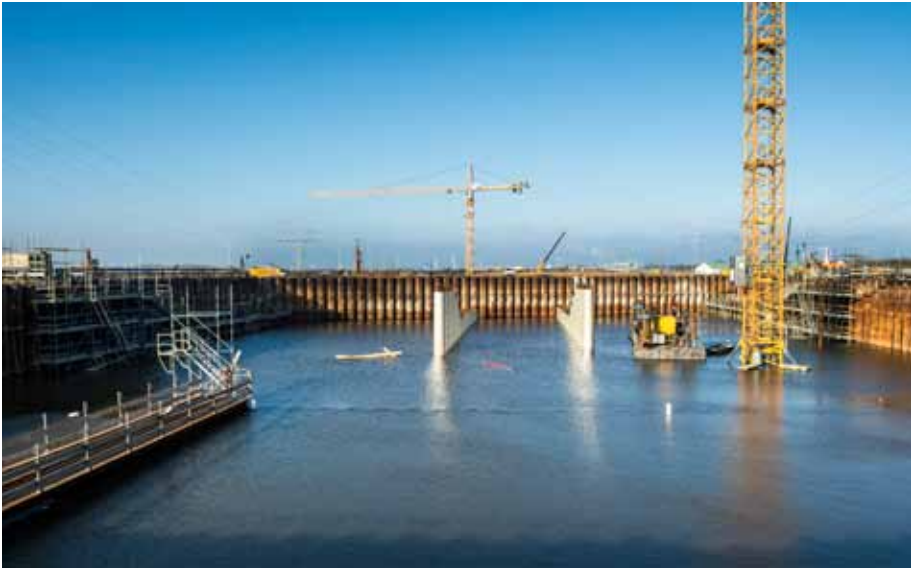
Figure 6.8: Water in the excavation site for the aqueduct near Muiden (Photo: Rijkswaterstaat)
